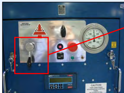
Purge & Leak Test Set
